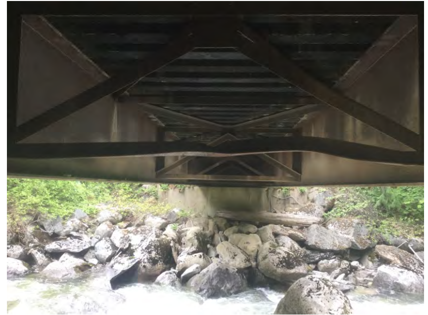
Damage to bottom chord
